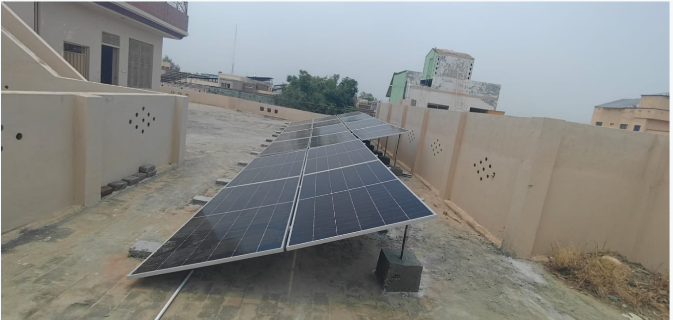
ROOFTOP PV DEPLOYMENT
